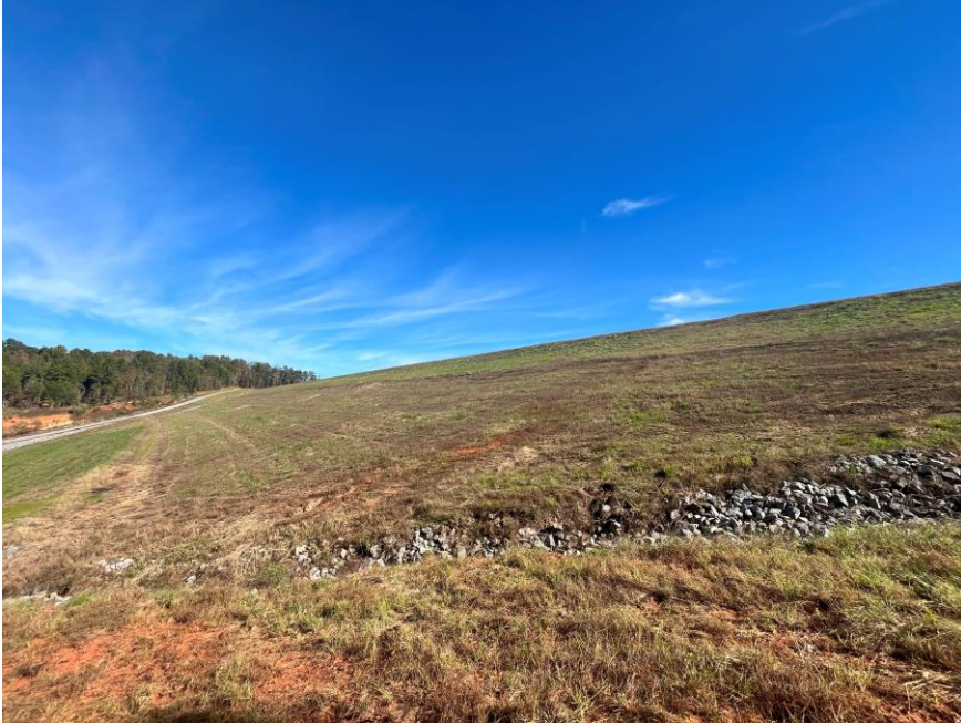
Photo 51. Field map number 13 facing East towards the CRWTP parcel. The rocks make up a drainage ditch.
